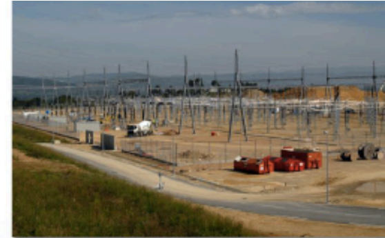
The ITER switchyard substation was energized in June 2012.
