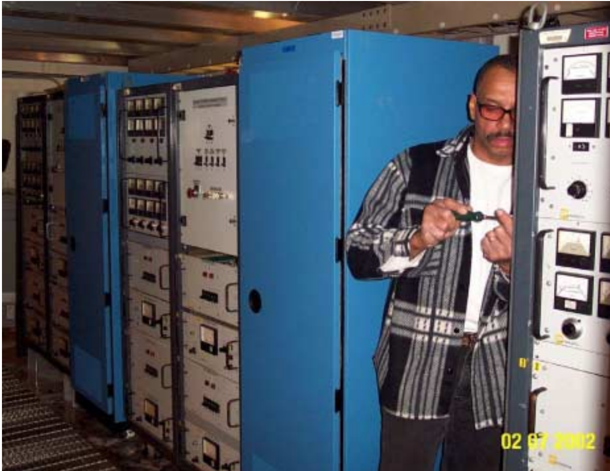
Figure 3.1-2. Installation of the Lower Hybrid transmitter protection and control racks. These racks are installed below the klystron mezzanine and the installation of cabling between the racks and the klystron carts is underway.
