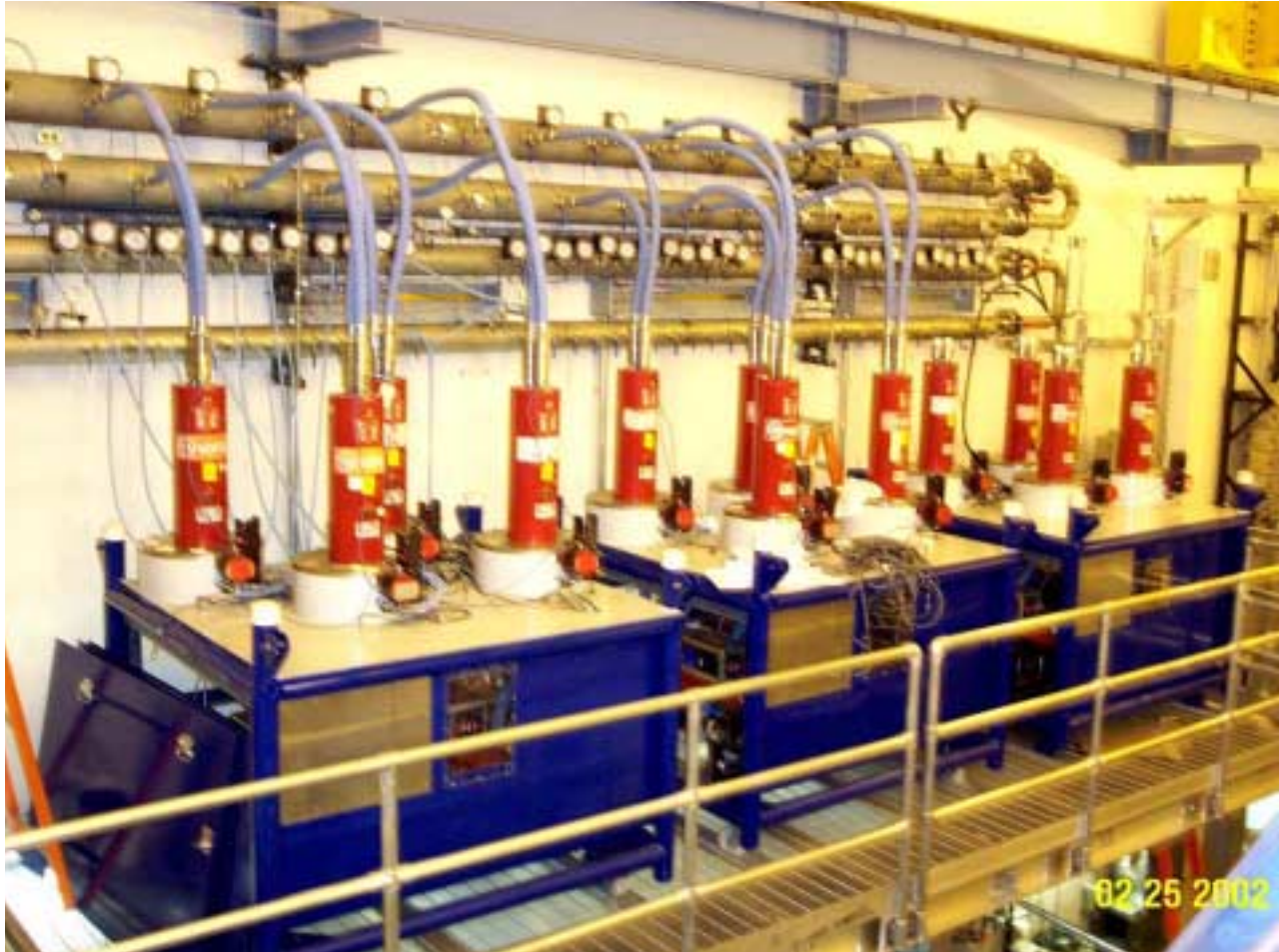
Figure 3.1-1. Installation of Lower Hybrid klystrons and carts on the new mezzanine. The water cooling system for the klystrons is also shown that will provide up to 1200 gallons/minute of cooling water to the tubes and other LH components.
