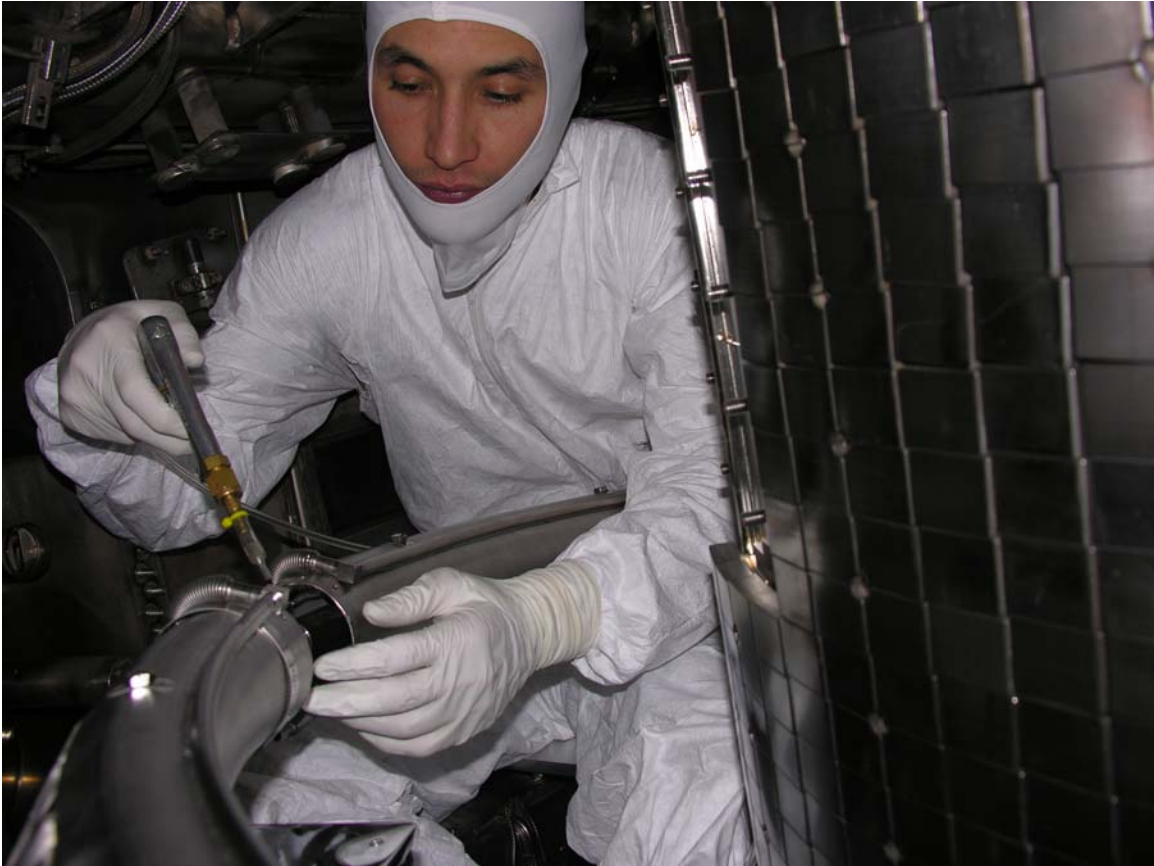
Figure 11.5. A view of the upper cryopump during installation. The liquid nitrogen shield is shown along with some of the liquid nitrogen feeds. Bellows in the feed-lines allow the cryopump to be assembled from three sections that can be passed through ports separately.
