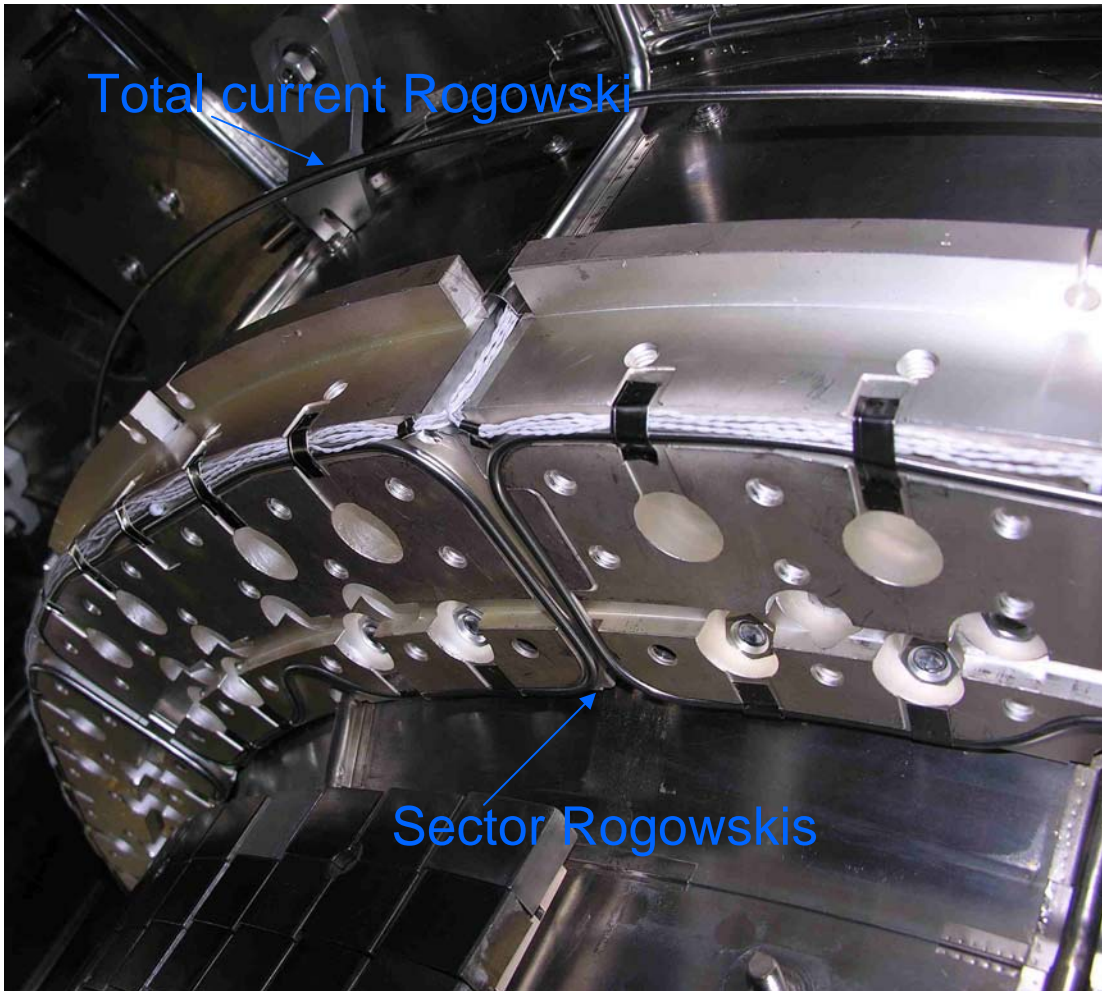
Figure 3.2.5 New Rogowski coils installed in the upper chamber.
